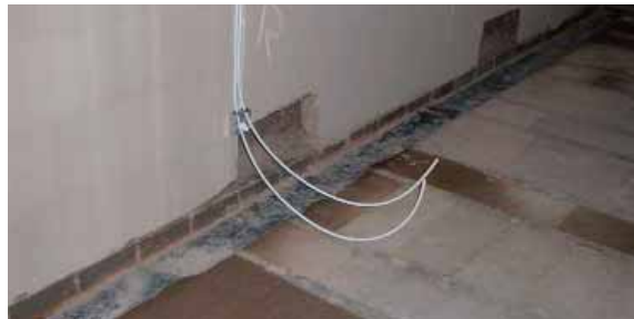
Figure 5: Blocks carefully removed to allow cavity to be cleared of excess mortar and debris
